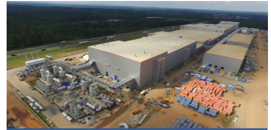
SK Innovations EV battery facility in Commerce, GA
